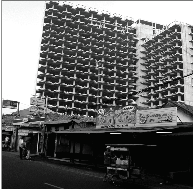
Work on Kemanggis Residence, in West Jakarta, one of the 1,000 Towers, was halted (photo courtesy of Suryono Herlambang)
